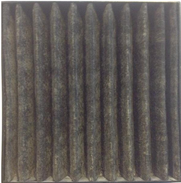
Dirty air filter – must be replaced
